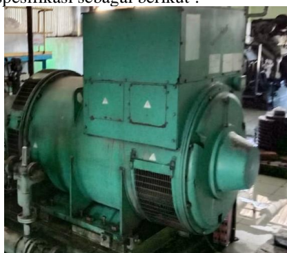
Gambar 7 Generator turbin uap
